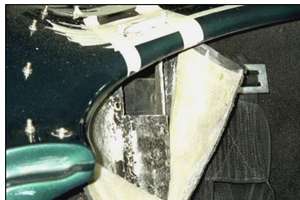
The location of the hole was marked on the masking tape and the hole in the deck drilled. The carpet was pulled back and a hole cut in the bulkhead.
